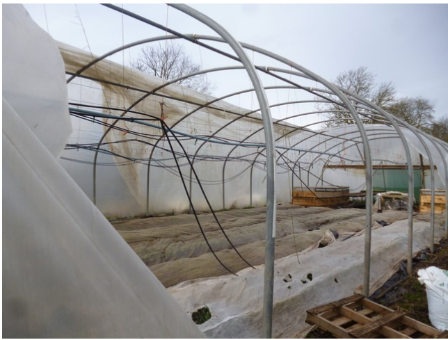
Damage caused to polytunnel 5 by storm Doris
